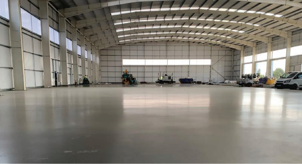
Fibre-suppressant dry-shake floor using PICS cure and seal. (Photo: Malin Industrial Concrete Floors Ltd.)
